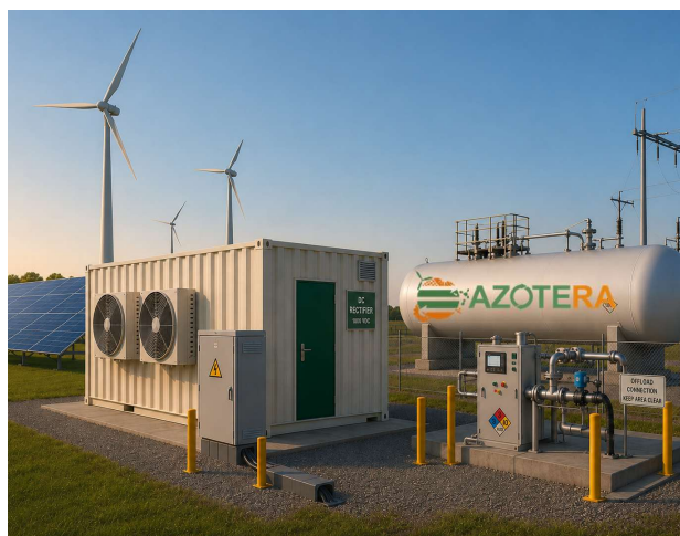
Figure 1. Azotera's energy solution combining distributed ammonia production with reliable backup generation
